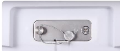
Locked with Wire Seal
